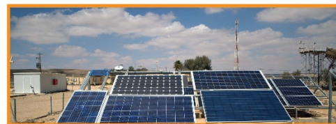
Solar panels capture energy from sunlight.
